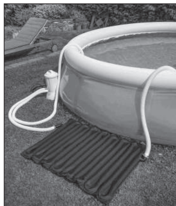
Solar Pool Water Heating
